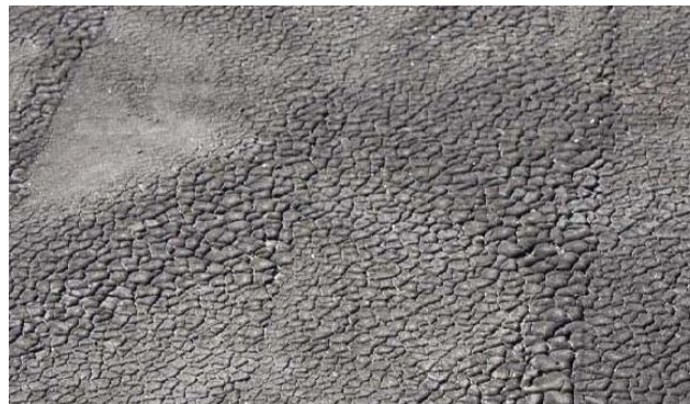
Alligating of Coal Tar Pitch Roof
