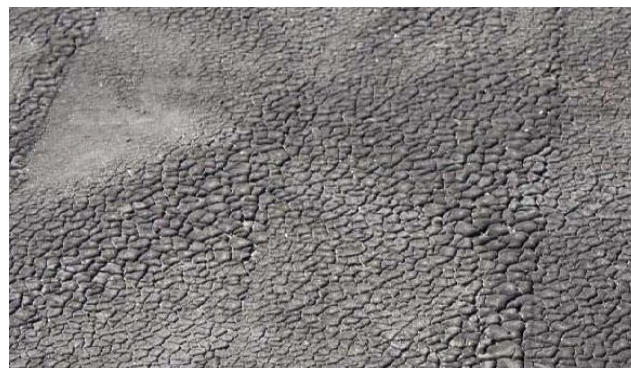
Alligating of Modified Bitumen Roof
